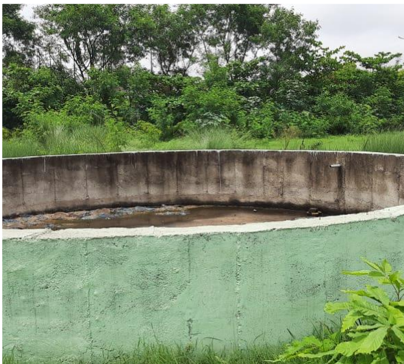
Rain water storage tanks
