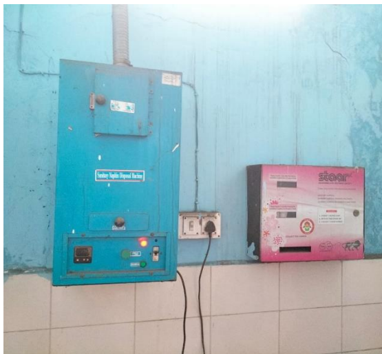
Incinerators for Sanitary pads disposal
